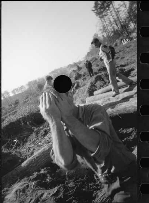
Transients building a bridge, Prince George's County, MD; photo by Carl Mydans, Nov. 1935.
